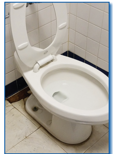
One of the bathrooms that floor tiles need replacement.
