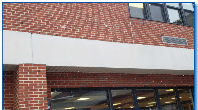
A picture of the EIFS system that needs repair.
